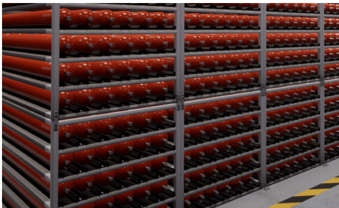
EnerVenue, an East West Bank client, is redefining battery storage and enhancing the future of clean energy.
